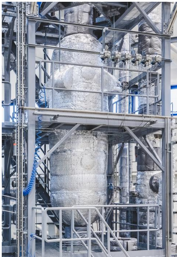
Figure 2-3: Primary heat exchanger of S-Allegro facility (installed)
